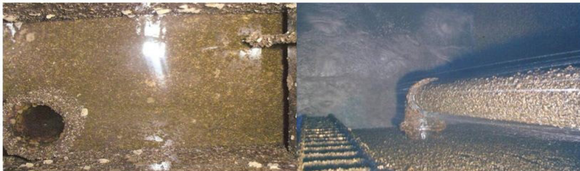
Figure 1. Zebra mussel infestation in raw water chambers at Sligo drinking water plant (photograph by Eamon Fox).
